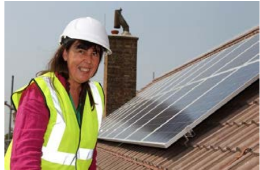
Cllr. Liz Wakefield inspecting installation of new solar panels on council homes.
