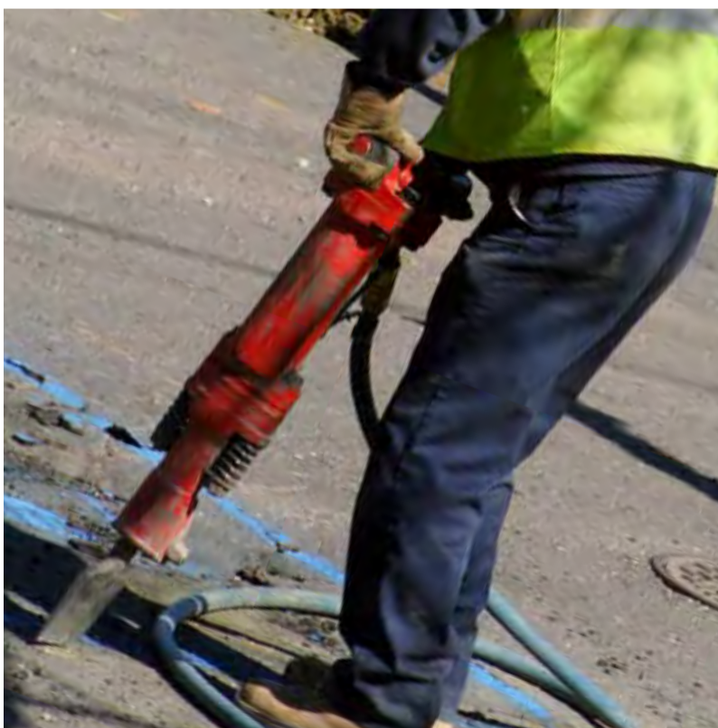
Cycle lane dig up! The Tory council is cutting jobs and services – and spending £1.1m removing existing cycle lanes from Grand Avenue
